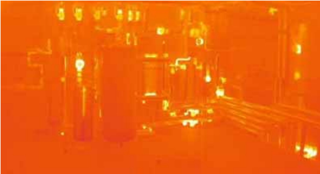
Fig.4: Thermographical recording of the technical room
