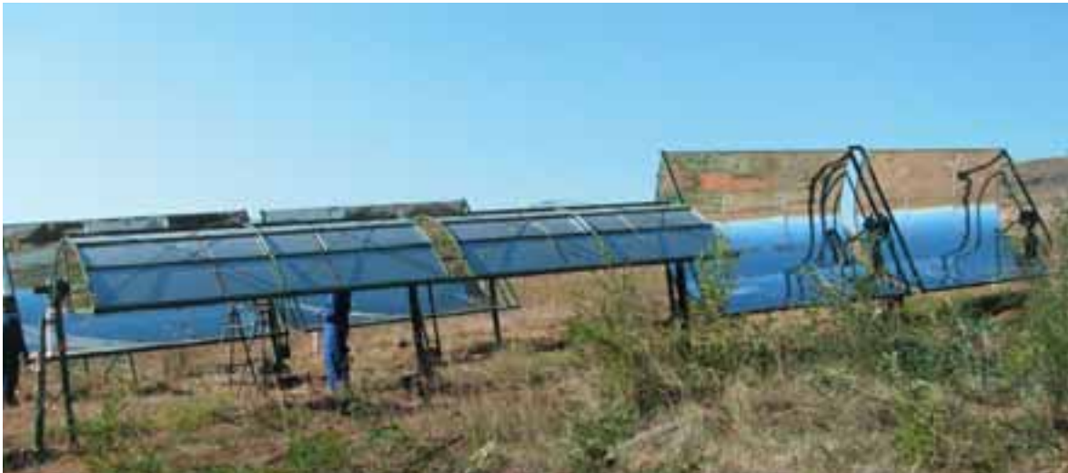
Figure 3: Prototype 3kWe Solar ORC in Lesotho, southern Africa, with a 75m 2 40x parabolic trough collector array.
