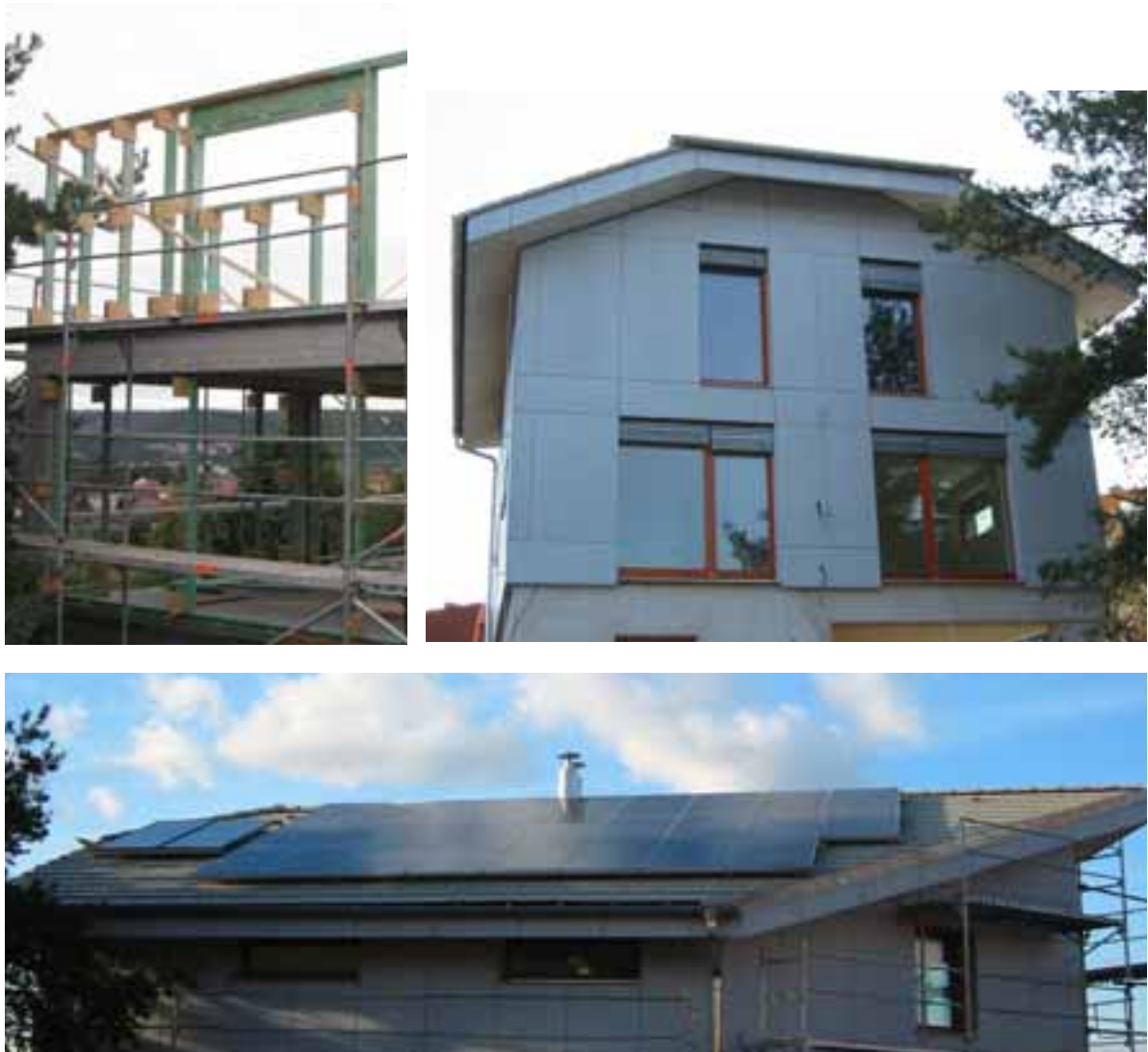
Fig. 1 House T – passive family house with combined structure (prefabricated concrete + wooden elements) can be described as a zero-energy house. The house is equipped with solar thermal system (4 m 2 ) and photovoltaic system (5,77 kWp) on the southern part of the roof. This house is a subject of monitoring and further studies. (Design: Tywoniak at al., 2008)
