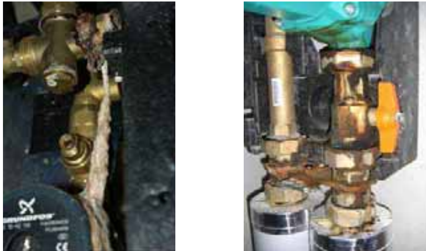
Fig. 6: Exemplarily illustration of located leakages in assembled hydraulic stations and pump groups
