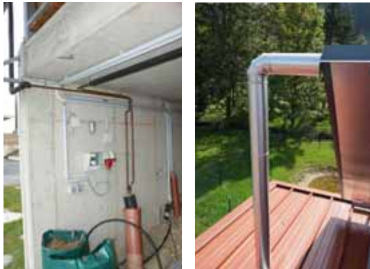
Fig. 10. External pipes insulated only partly (left), correct protection against UV-rays and animal bites (right)
