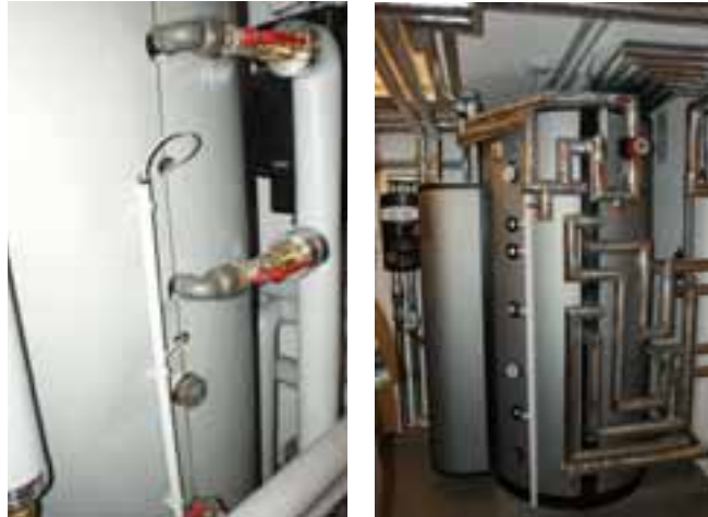
Fig. 6. Heat storage tank connections are not insulated (left), storage tank with exemplary good thermosiphon heat trap installation of the pipe connection (right)
