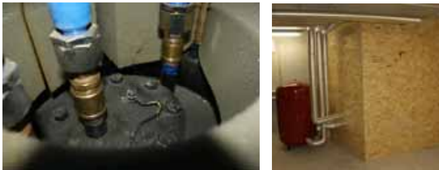
Fig. 5. Very poor heat storage insulation at the top of a tank (left), good alternative of heat storage insulation, on site build box filled with cellulose insulation material (right)
