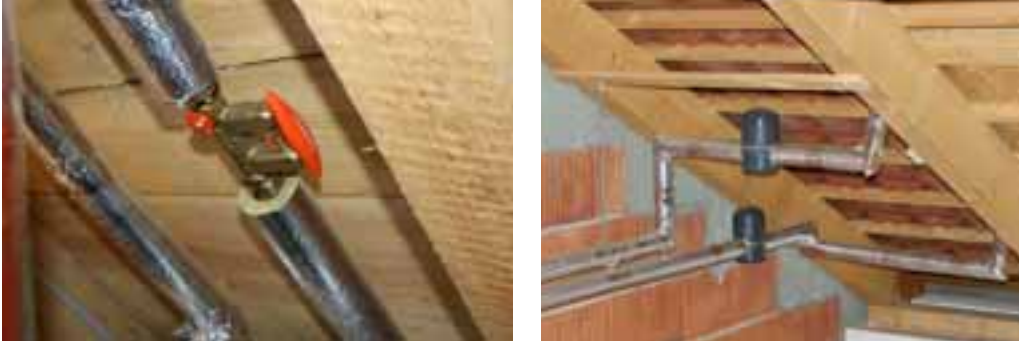
Fig. 9. Not temperature resistant flow regulation valve within high temperature critical parts of the collector loop (left), correct manual deaeration valves within high quality insulation (right)
