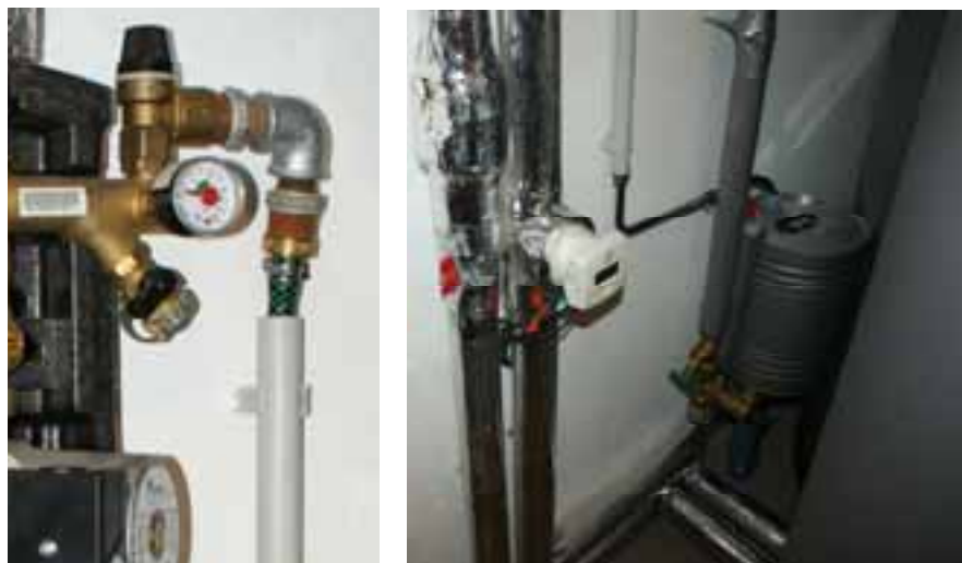
Fig. 8. Drain pipe not temperature resistant (left), temperature resistant collection vessel, made of metal (right)
