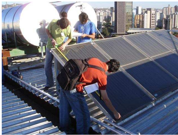
Fig. 3. Detail of the solar collector shadowed by a battery ahead. Source: GREEN Archives
