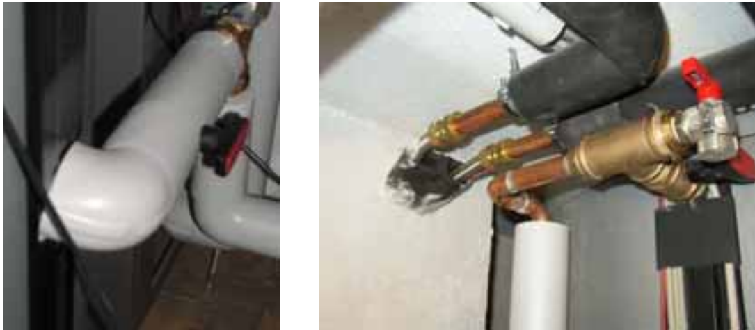
Fig. 3. Insulation of the heat store connections, well done (left side) and missing (right side)
