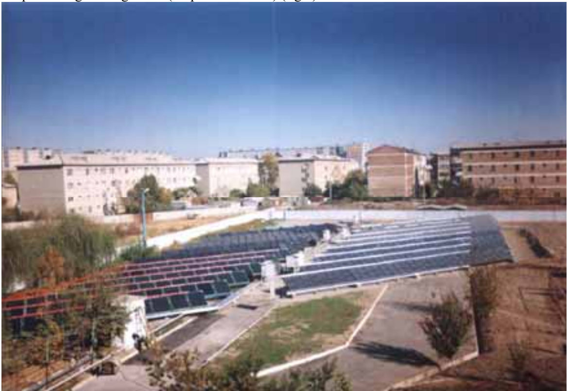
Fig.1. Field of the solar collectors working together with a boiler-house in the district "Vodnik". This project has been executed at support of program TACIS (2003).
