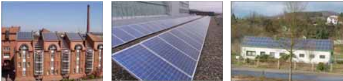
Fig. 2. By solarcampus initiated installation of three photovoltaic systems on university's roofs.
