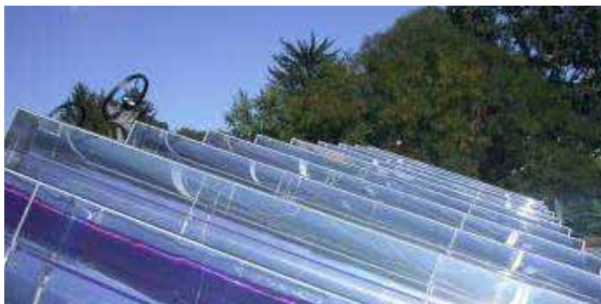
Fig. 8. 10 parabolic trough collectors at the test facility in Gleisdorf.
