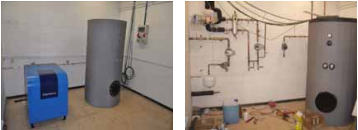
Fig. 3. Air conditioning solar plant. Technical room (in progress). Left: SorTech ACS 08 Adsorption chiller and buffer. Right: Buffer and hydraulics.
