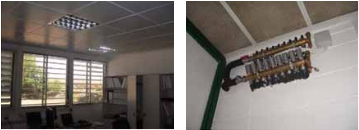
Fig. 2. Air conditioning solar plant. Left: radiant ceiling. Right: radiant ceiling distribution kit.
