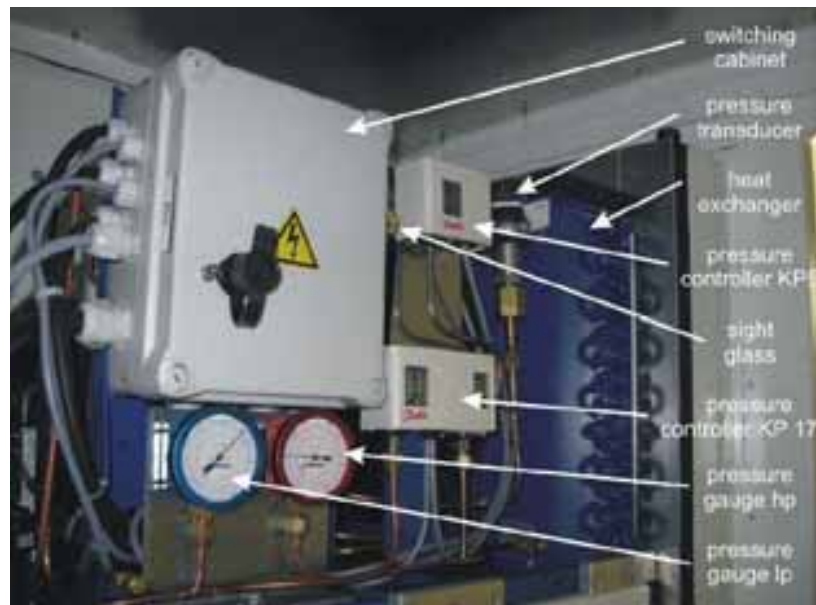
Fig. 5: Cooling unit front view
