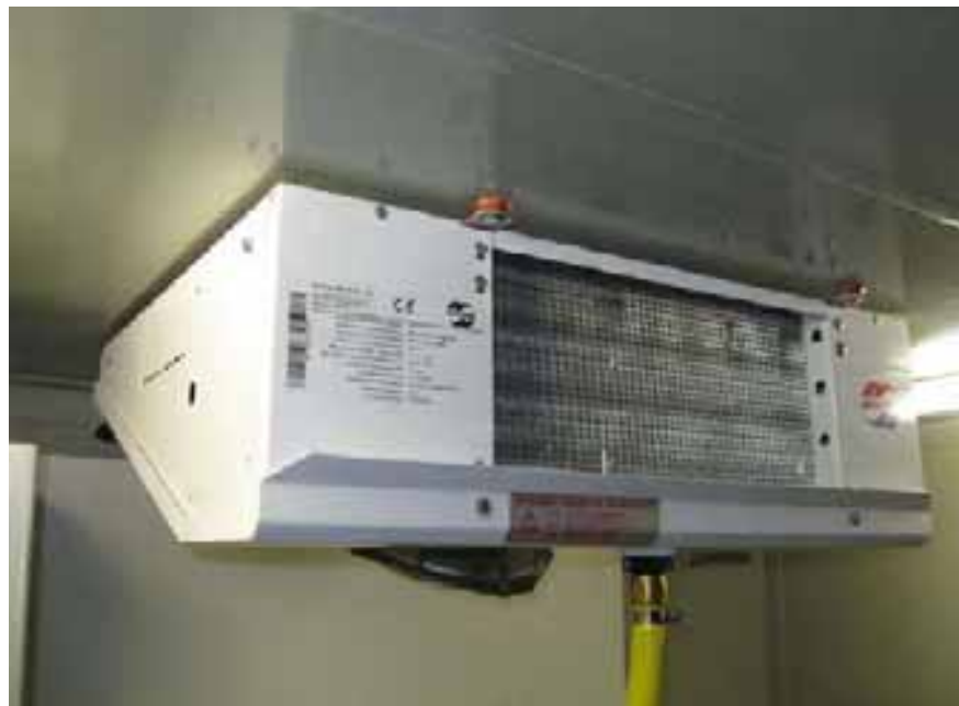
Fig. 6: Evaporator inside the shelter
