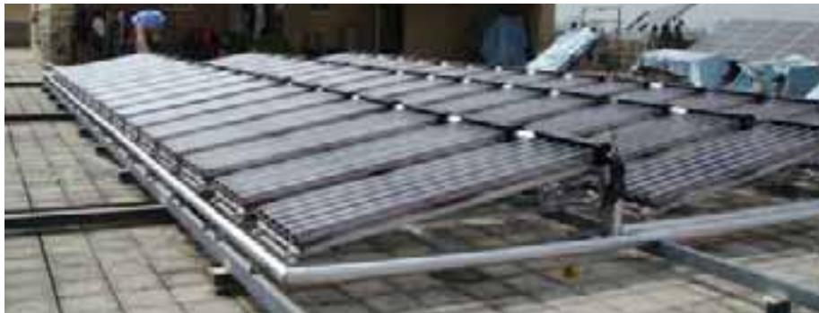
Figure 6 Solar heating system of SACH-2.
