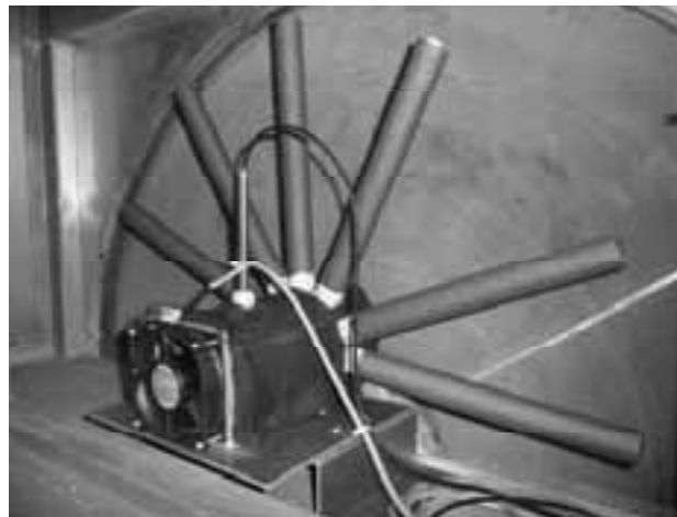
Fig. 3: Measurement device downstream the desiccant wheel in the return air duct
