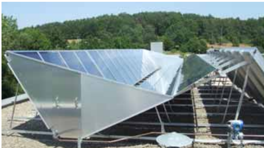
Fig. 6: RefleC-collector field at laundry "Laguna" in Marburg, Germany under construction. Due to the risk of glare and radiation concentration in the ambient, the ends of the trough were equipped with vertical metal sheets.
