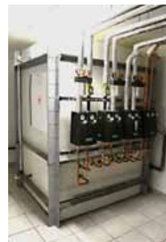
Fig. 7. Installation of the FLEXSAVE heat storage of FSAVE Solartechnik GmbH.
