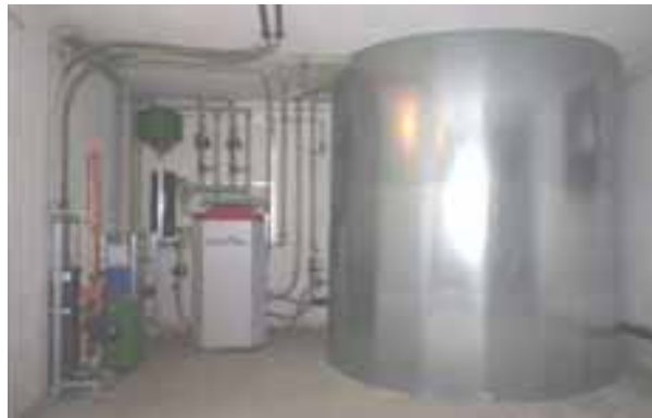
Figure 6: Heat pump and buffer storage tank (Source: AEE INTEC)
