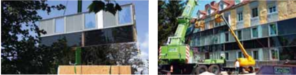
Figure 5: Assembling of façade modules with integrated solar thermal collectors (Source: AEE INTEC)
