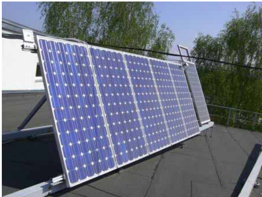
Fig. 7. PV batteries of the quasi-autonomous system
