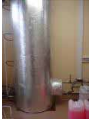
Fig. 4. Hot water accumulator
