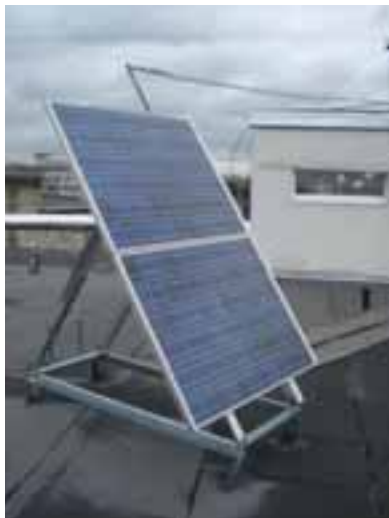
Fig. 5. PV batteries of the autonomous system
