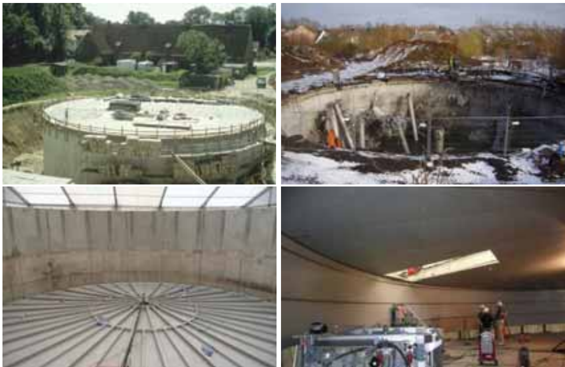
Fig. 4: STES in Hamburg during construction in 1996 (left) and reconstruction in 2010 (upper right and bottom)
