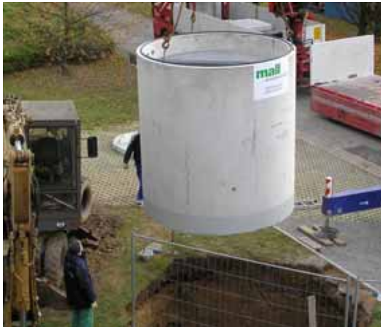
Fig. 1: Installation of the first storage tank test sample at the ISFH test area. Outer height 3.15 m, outer diameter 2.74 m, water volume 5.5 m 3
