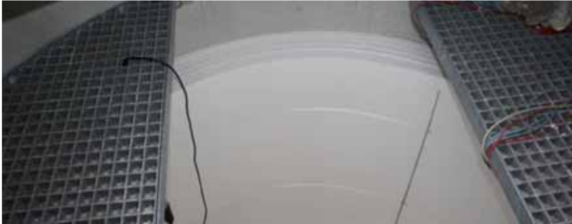
Fig. 3: Built-in and clamped XPS panels of the prototypes storage jacket. The insulation of the mantle consists of 6 panel layers forming an overall thickness of 18 cm.
