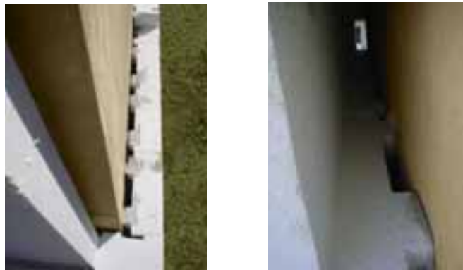
Fig. 3. Pictures of an installation of a test wall at Ing. Kleebinder Ges.m.b.H.
