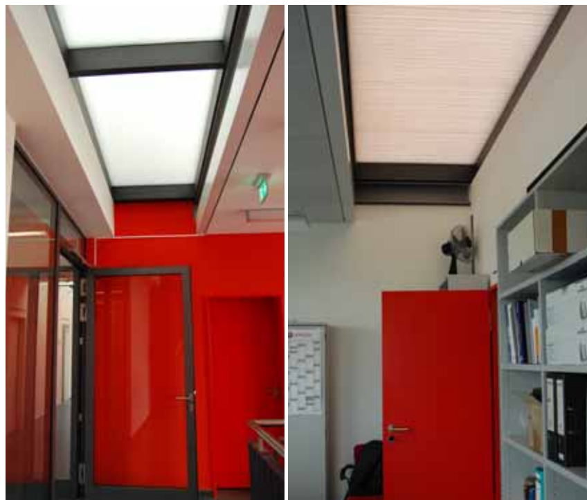
Fig. 3: Translucent aerogel glazing in the stairways (left); Aerogel-filled double skin sheets in the office rooms (right).
