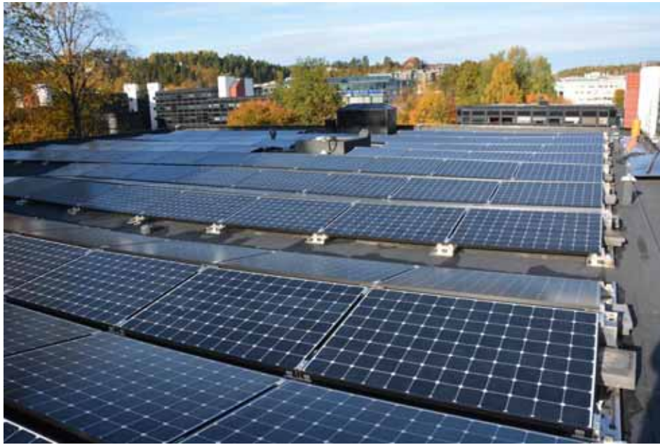
Figure 6: PV-system consisting of Sunpower E20 modules and Knubix EW mounting System.
