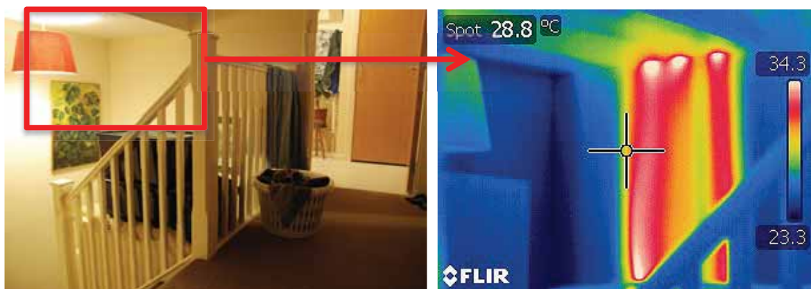
Fig. 10: Left: view of the stairwell and right: thermographic image of boxed area showing uninsulated hot water pipes running within.
