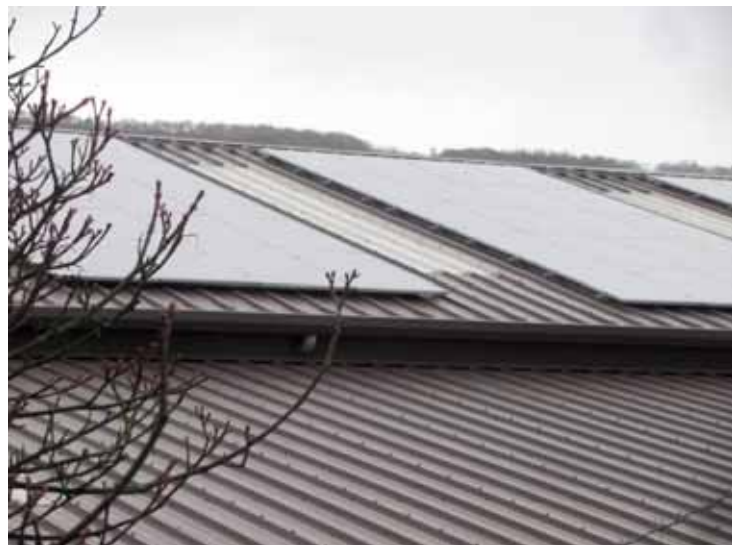
Figure 4: Building added PVs mounted either side of roof lights on roof of Muir Group HQ, Inverkeithing, Fife. Roofscape is visible from the road (position of the photographer).
