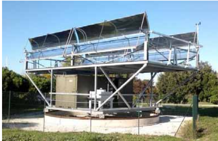
Figure 2: Outside view of the micro CHP system.
