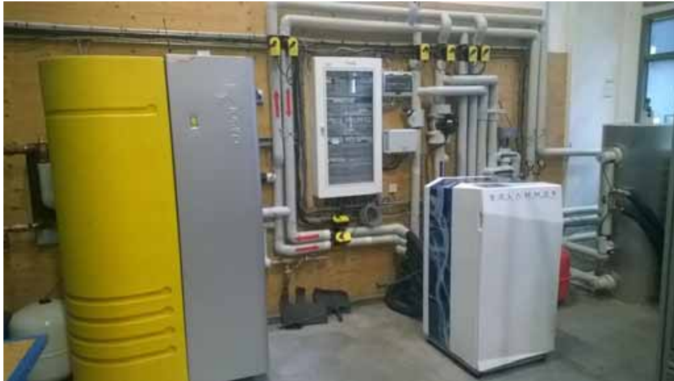
Fig 10: View of operating installation
