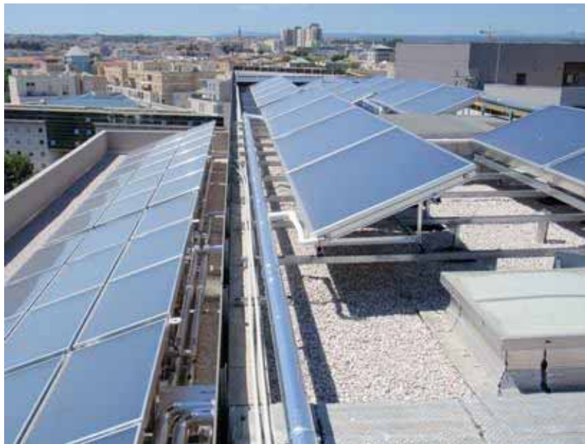
Figure 3. Partial view of solar collector field (double glazed flat plate collectors)
