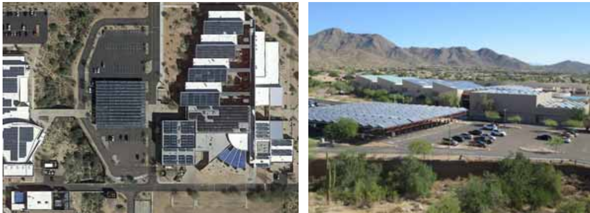
Fig. 1: Overview collector fields from Google Maps (© www.google.com) and from a terrestrial photograph (© www.solid.at)
