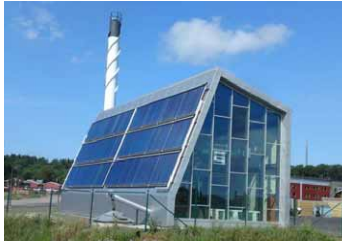
Fig. 1: Heating plant with evacuated tube solar collectors
