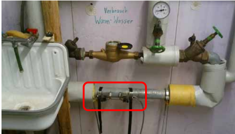
Fig. 4: Logging of the hot water consumption at a substation
