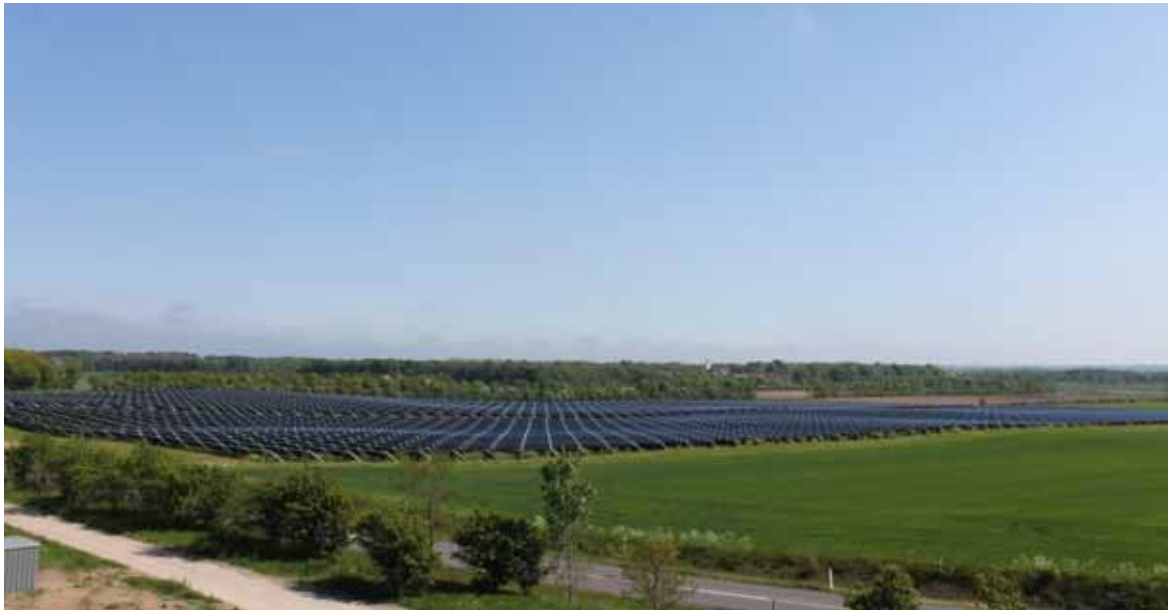
Fig. 2. Dronninglund solar heating plant with a collector area of 37573 m 2 installed 2014.
