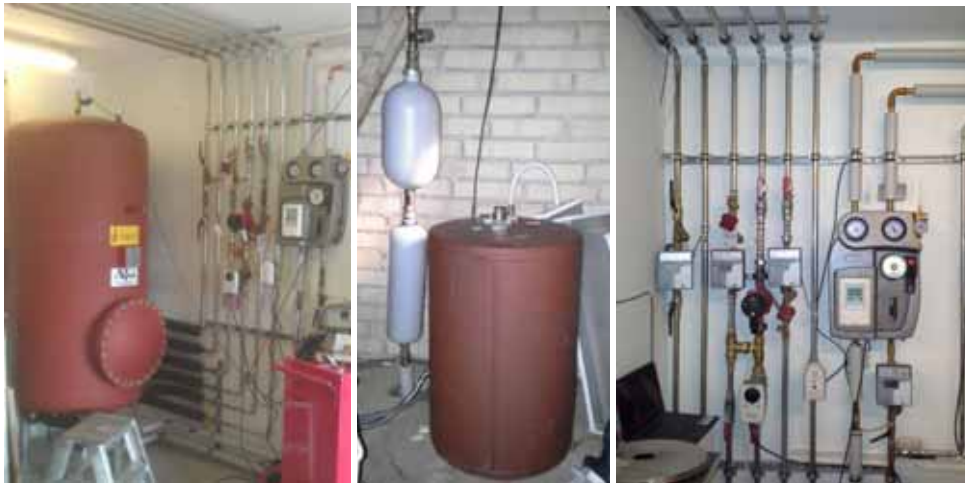
Figure 2c: Some more pictures from the demonstration system in Sorö, Denmark. The left picture is before insulation of the storage tank. Note in the middle picture the small drain back vessels (white) and the combined expansion tank (red). Note in the right picture, the pump unit that was convenient to use for the installer, but gave extra pressure drop and malfunction of the combined expansion vessel in the beginning.
