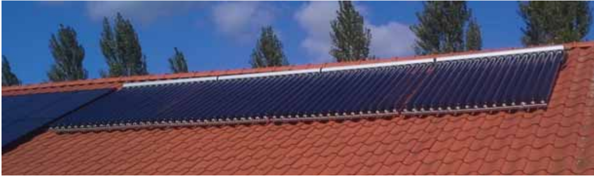
Figure 2a. Sunda Seido 5, Vacuum tube solar collectors, in the demo system . (The PV system seen to the far left only interacts with the electric grid.)
