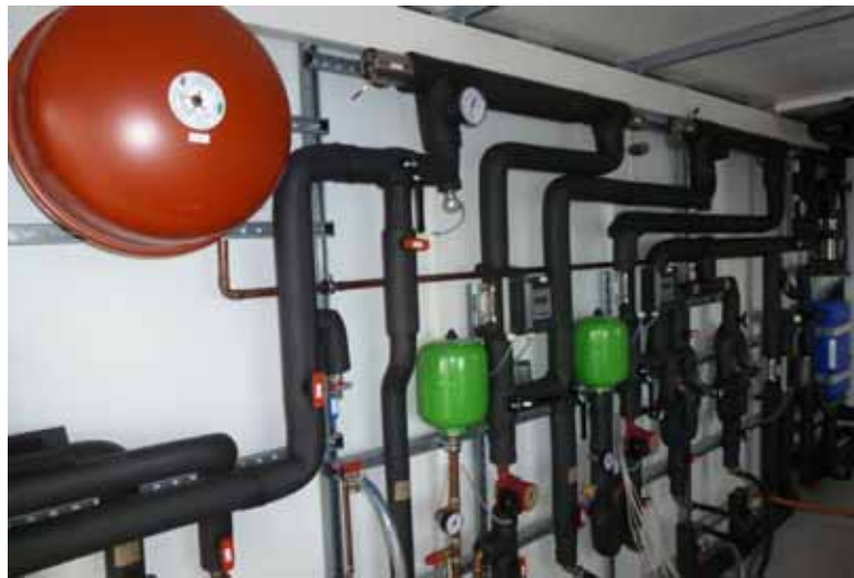
Figure 1: Hydraulics of the mobile all-in-one test facility (overview)
