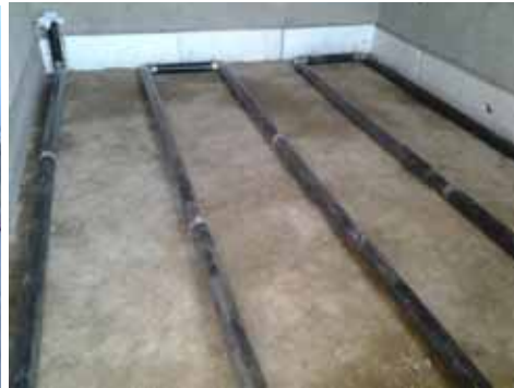
Fig. 4: The metal heat exchanger coil
