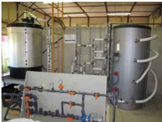
Fig.4 - Solar thermal desalination test facility to operate and testing solar desalination prototypes at LNEG laboratory.
