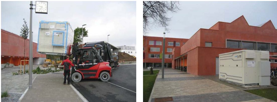
Fig. 8: Delivery and installed VR-battery
