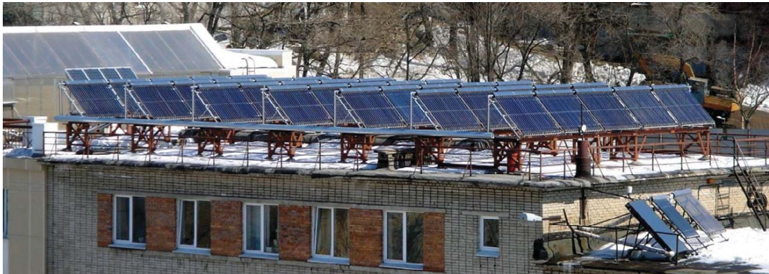
Fig. 12: Experimental solar installation of hot water and heating.
