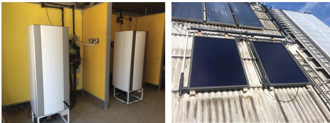
Fig. 2 Pictures of the storage tanks and solar collectors in the two SDHW systems.
