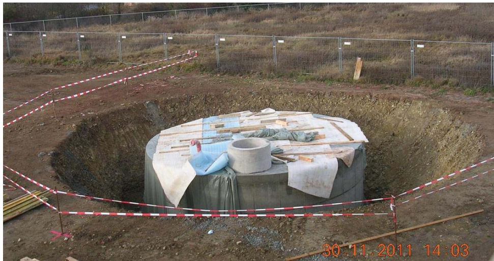
Fig. 2: Underground fire protection water tank.
