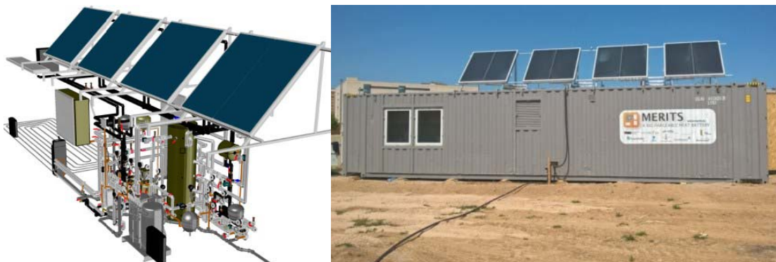
Fig. 1: MERITS Field Test Demonstrator 3D systems model (left) and Field Test Demonstration container during pre-testing in Lleida, Spain (right)
