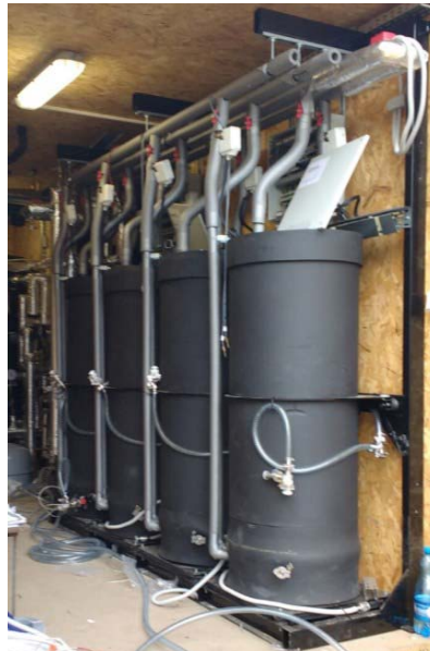
Fig. 4: Rack with 4 thermochemical storage modules inside the Field Test Demonstrator
