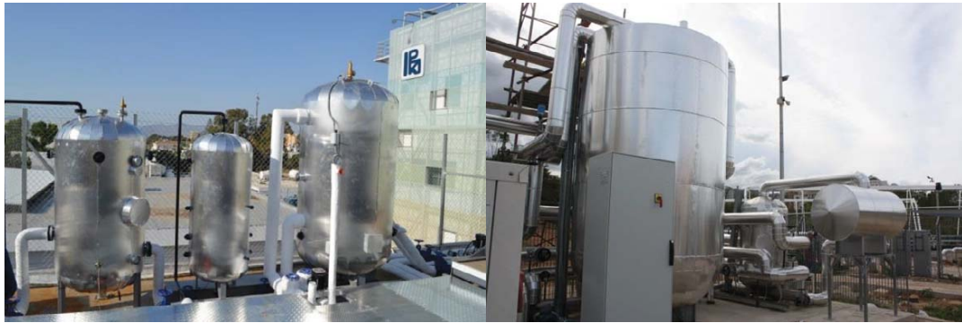
Figure 9. Buffer of oil, expansion vessel, thermal storage tank (left to right) at CyI (left) and molten salts storage, oil storage and expansion tank (left to right) at ARCA (right)
