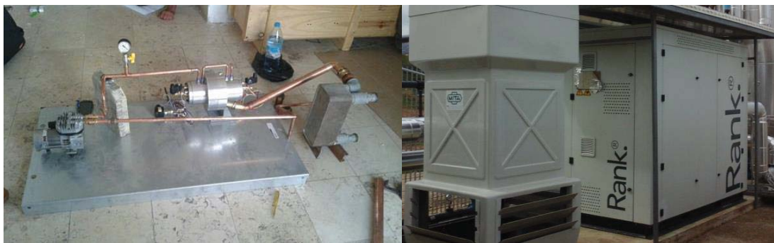
Figure 12. Steam turbine during the installation in Irbid (left) and ORC Rank turbine in Palermo with cooling tower (right)
