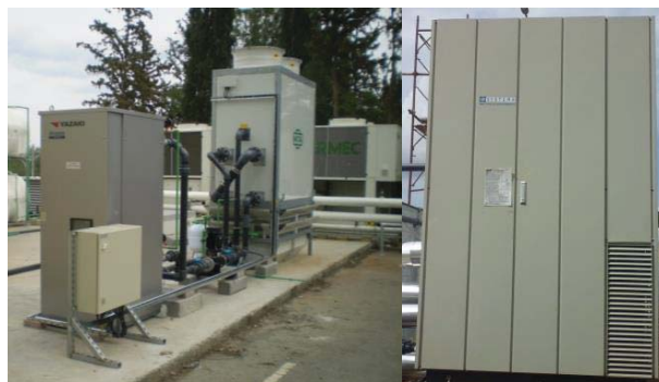
Figure 11. Absorption chiller and cooling tower at CyI (left) and at ARCA (right)
