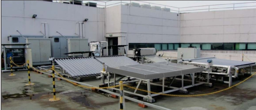
Fig. 1: Solar Thermal collector testing system at the roof top of the Solar Energy Research Institute of Singapore (SERIS). Three different solar thermal collectors were installed for the test operation.
