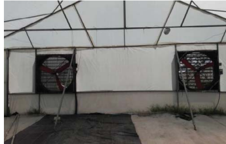
Fig. 10. Fans in opposite face to evaporative pad.
