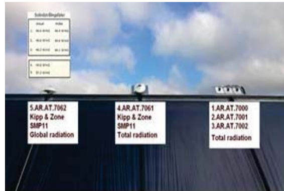
Fig.3. Pyranometers in the middle of flat plate collector field
