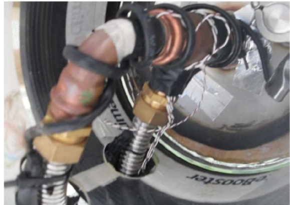
Fig. 14: Electrical tracer to the inlet and outlet pipe of the module.
