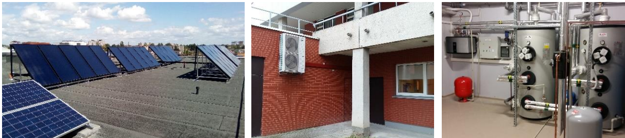
Fig. 1: View of combined ST and HP system in one of the hospitals.
