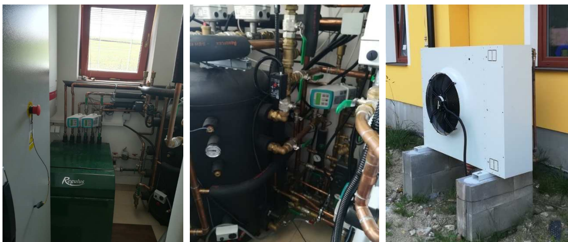
Fig. 7: Heat pump, storage tanks and external air unit for heat pump
