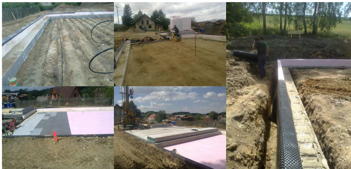
Fig. 2: Realization of simple and low cost ground seasonal storage
