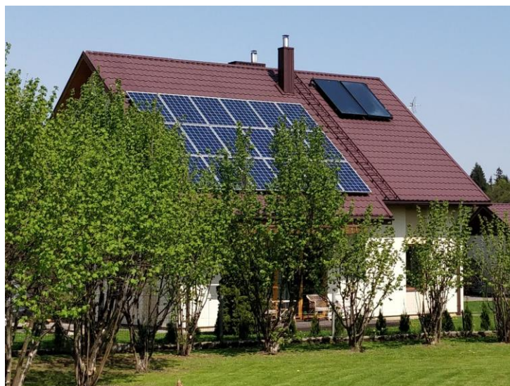
Fig. 1: Single family house with ST (5m 2 ) and PV (5kWp) systems.
