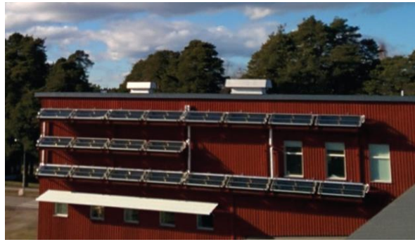
Fig. 4. Wall facade installation of asymmetric C-PVT solar collector prototypes at Gävle University, Sweden.
